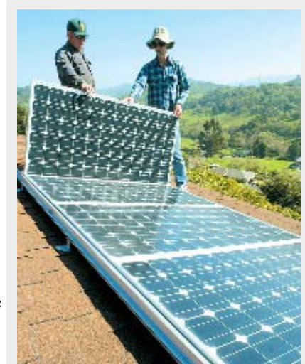
Kurt Newick and Bruce Gordon install solar panels on the roof of a Morgan Hill home.
